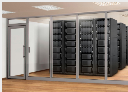
DATA CLOSET with racked workstations
